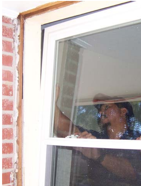
Contractor Tim McIntosh installs a new, energy efficient window to weatherize the home of a family of nine in Baton Rouge, LA.
